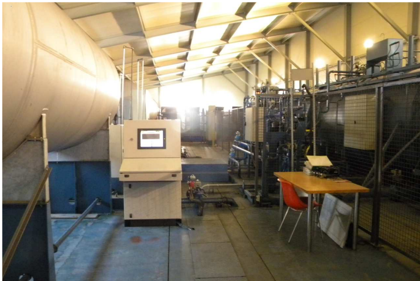
Figure 10 Wood impregnation plant. Chemical tanks are located on the left side of the picture. The pressure vessel is located on the right side of the picture.
